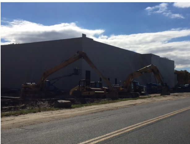
Above: Blount Fine Foods is adding 50,000 s/f to their Fall River facility
