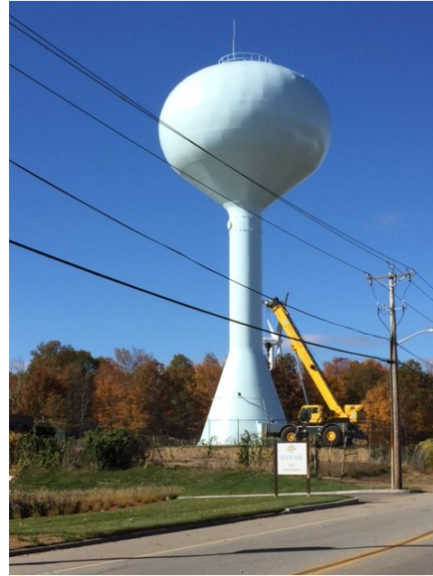
Left: The new $3.3 million, 750,000 gallon water tank located in the Fall River Industrial Park will increase water pressure for all business park tenants.
